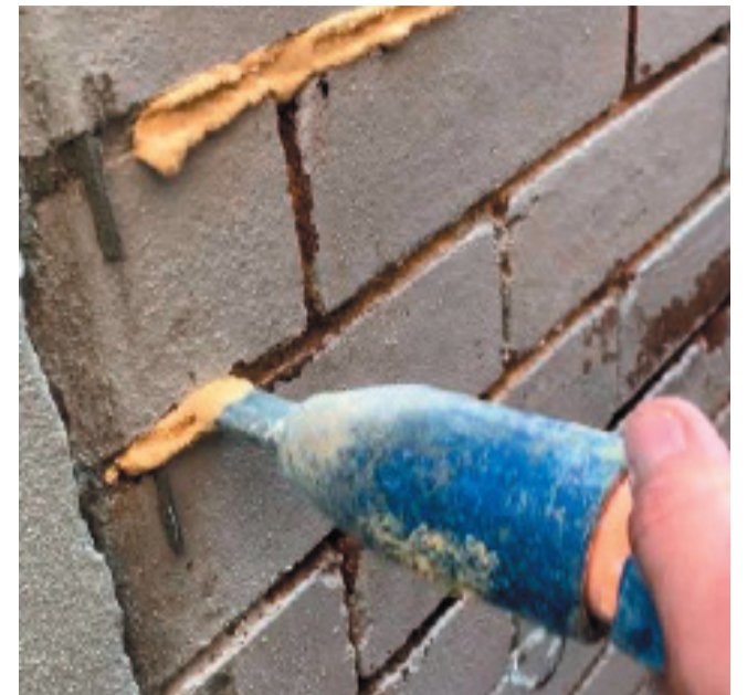
The new mortar should be applied with a mortar gun to ensure it fills the holes and not just fill the surface with a trowel.
